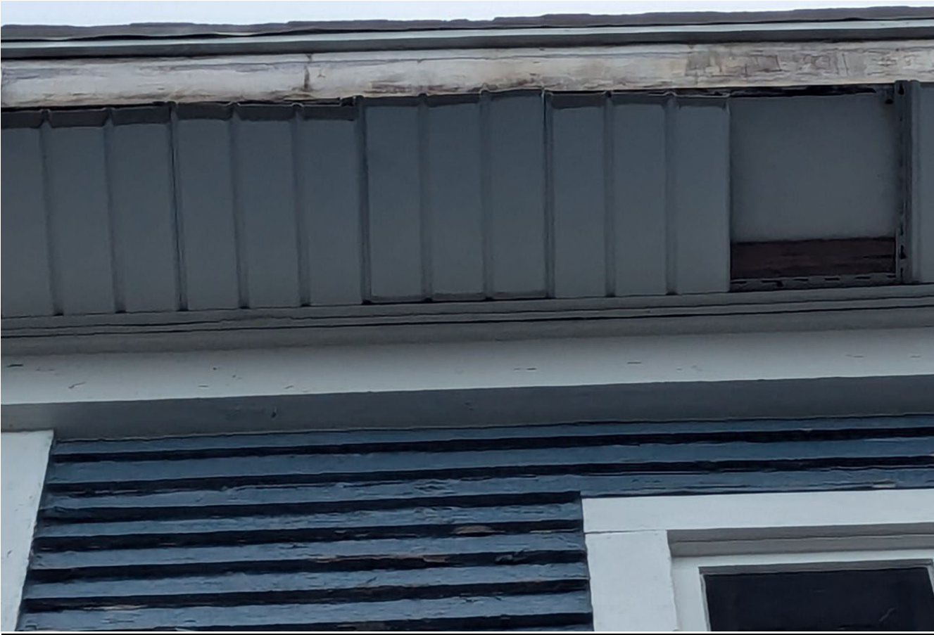
Siding wood rot, soffit/fascia damage
