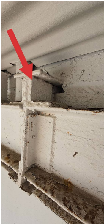
Beam passes through CMU block wall and is an attachment point for the steel I-beam ledger. Corrosion present. Recommend paint is removed and beam treated for corrosion.
