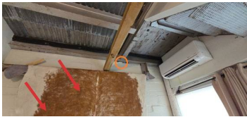
Orange- Steel I-beam rests on CMU block wall. Behind cow hide there is evidence of step cracking in the block wall and it has been repaired. Home was built in 1949 and some movement is expected.
