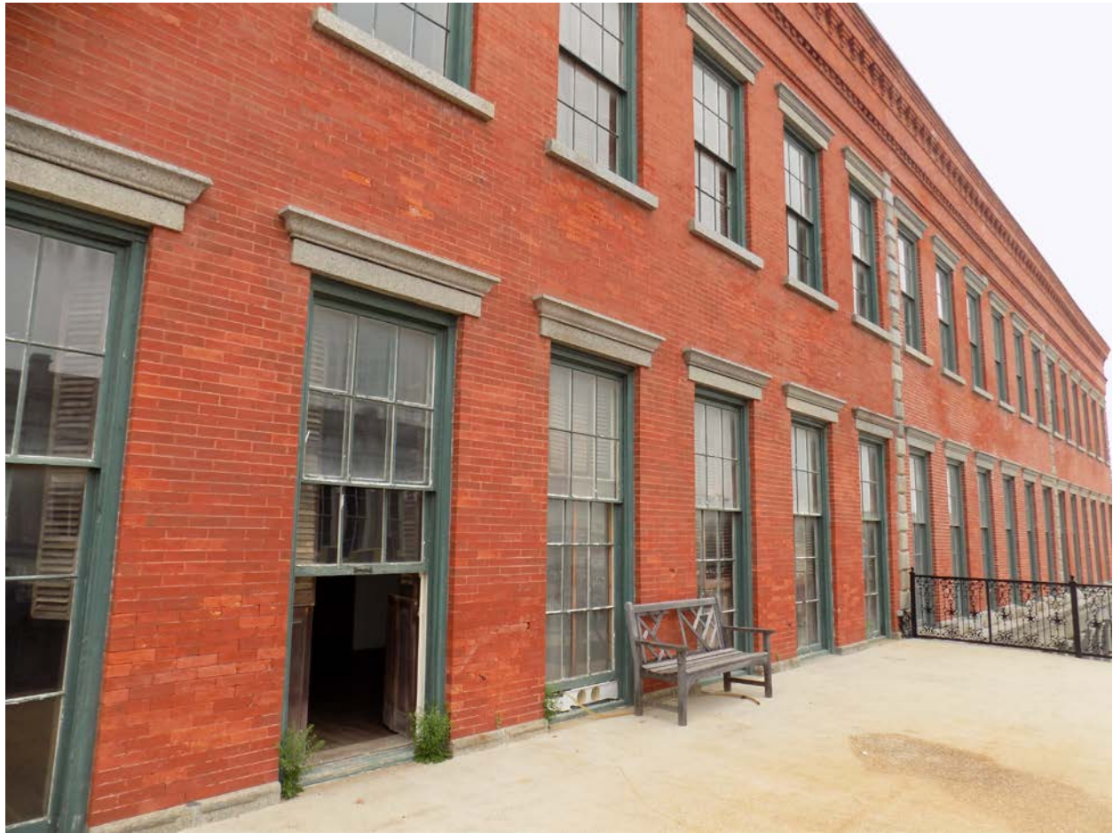
Photo 21: View of Exterior windows. Note: The glazing compound will be removed. Windows will be replaced. Broken or cracked glass will be replaced. Windows will be painted. (Typical for all windows on north and south elevations)
