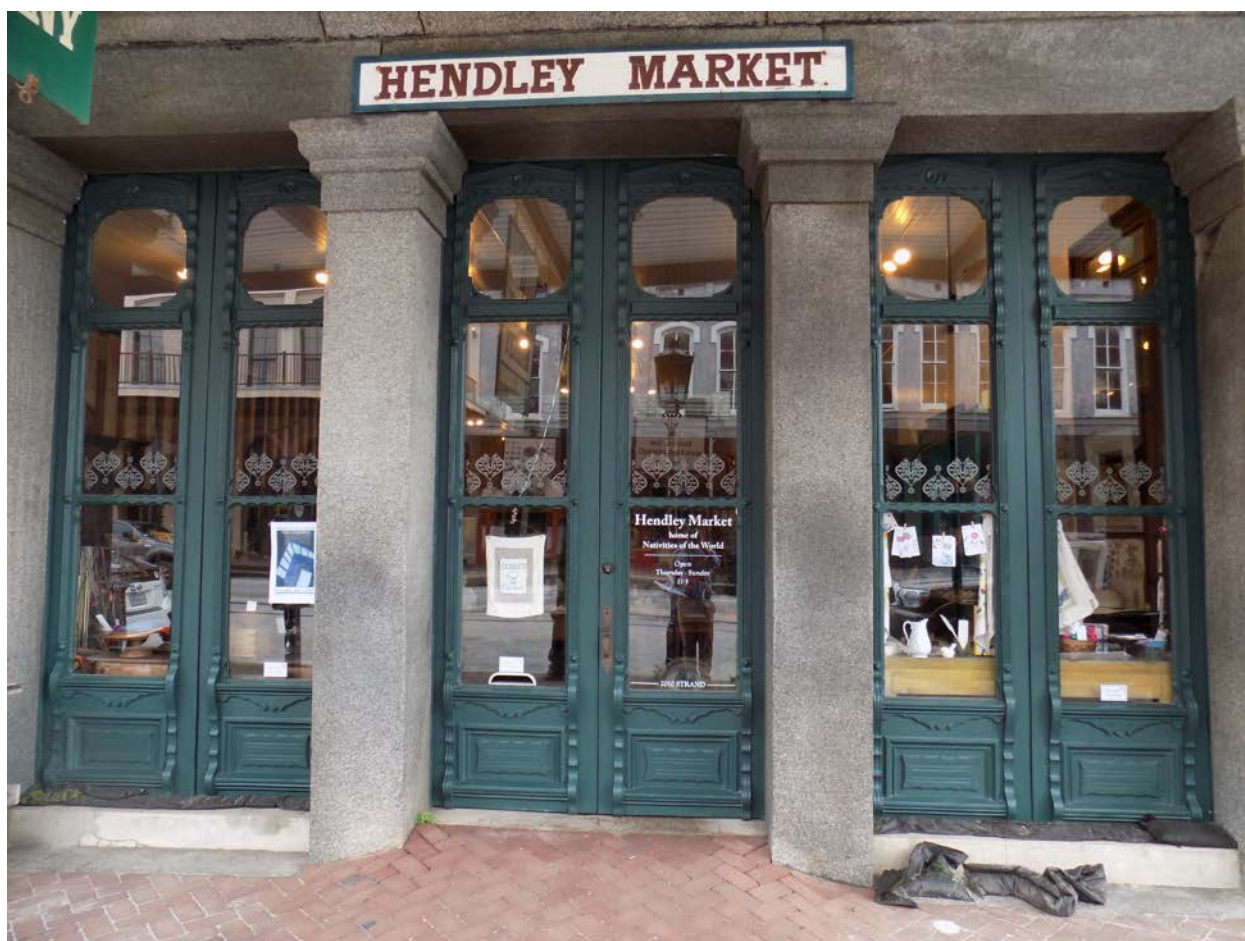
Photo 24: View of existing doors on Strand. Note: Doors were repaired to bring first floor mercantile to working condition.
