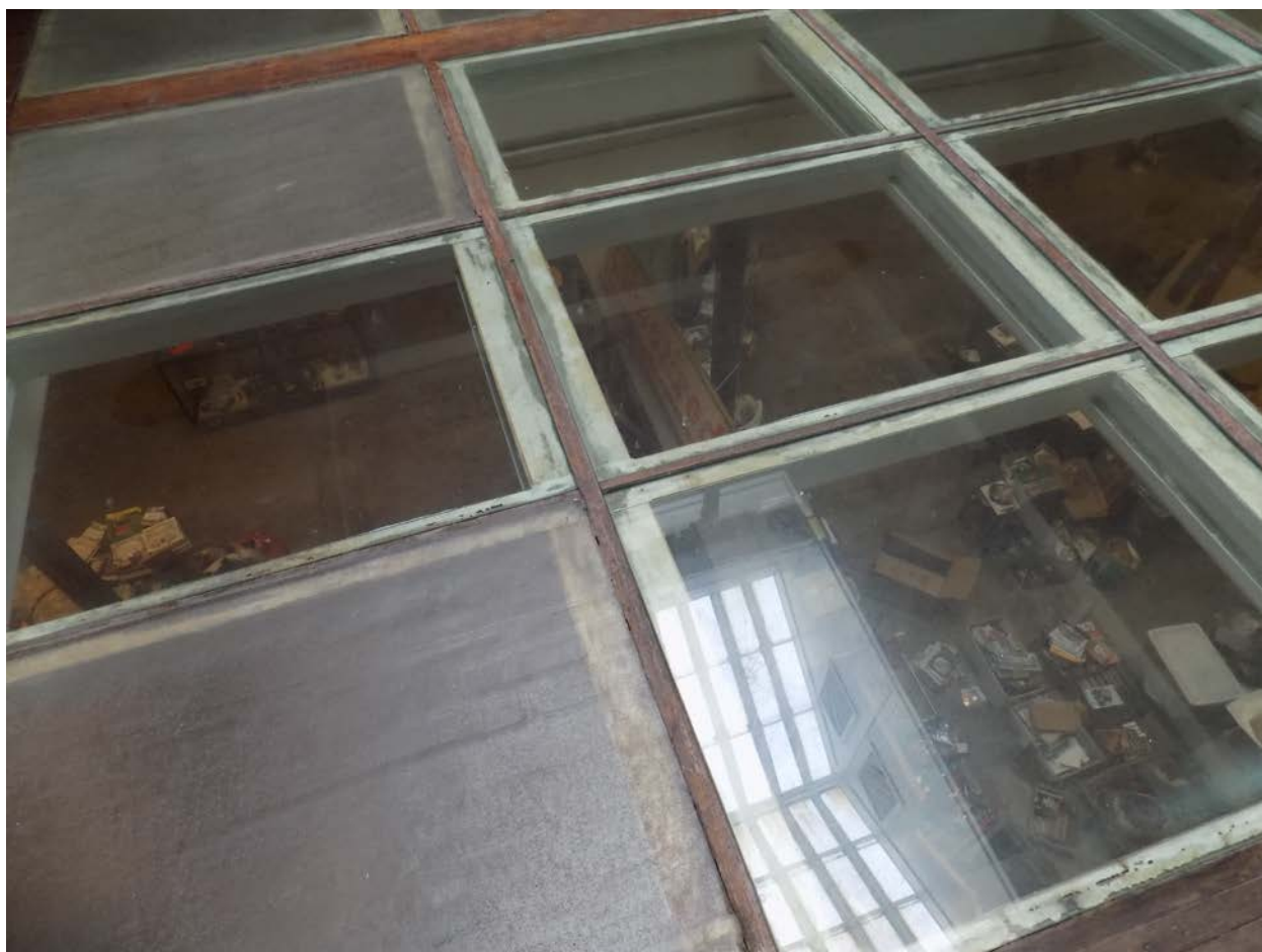
Photo 4: View of Glass atrium floor (note- original glass panels have a “sand” texture and replacement glass is clear). Note: Cracked replacement glass floor panels will be replaced. Historic original glass panels will be retained. Any cracks in historic panels will be address by adding additional supports from below. Support method will be developed by structural engineer on an individual case-by-case requirement.
