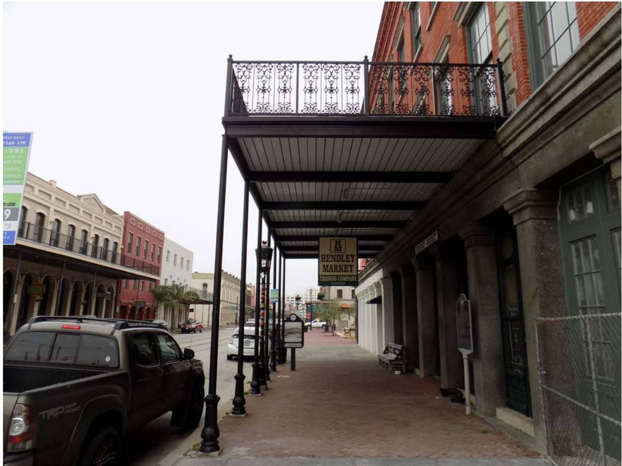
Photo 26: View of Existing sidewalk canopy/balcony was added around 2000. The steel support framing and railing were rusting. Note: Heavily rusted steel was removed and/oil cleaned. New steel stiffeners were continuously welded around the perimeter edge. The steel will be ground to bare metal and primed with zinc rich primer before painting. Sidewalk was a hazard and therefore was required to be completed as soon as possible.
