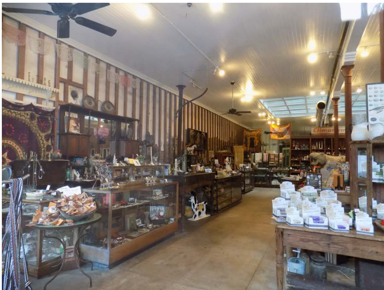
Photo 27: View of interior of Hendley Market, note the original cast iron interior column. It has developed a vertical split. There appears to have been a flaw in the original casting, and the 9 feet of floodwaters during Hurricane Ike has resulted in internal rusting splitting the column. The split has continued to grow since first observed. Note: The cast iron column is no longer structurally sound. It cannot be repaired to continue to function supporting the load of the two floors above. It will be removed and a steel pipe column installed to replace it.
